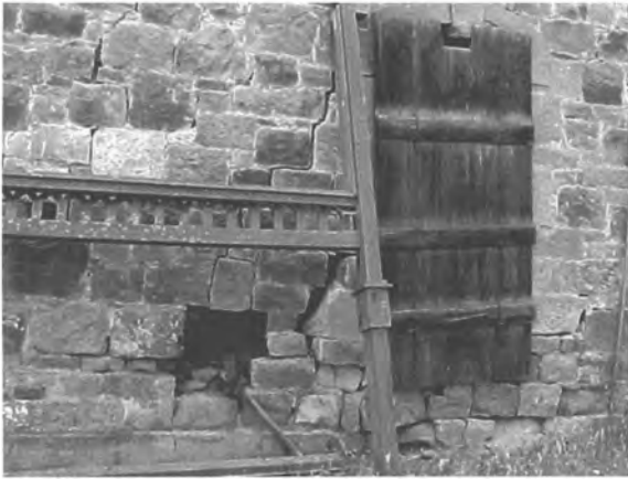
Crumbling wall of the John Marsh House in East Contra Costa County
