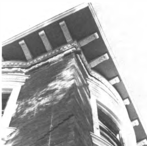
Look closely at "the brick", forced out by the earthquake and dangling, now, for 3 months near the top of the Santa Cruz Trust Building
