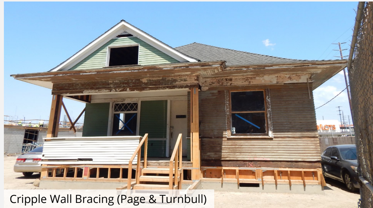
Foundation anchors (Structural Focus)
